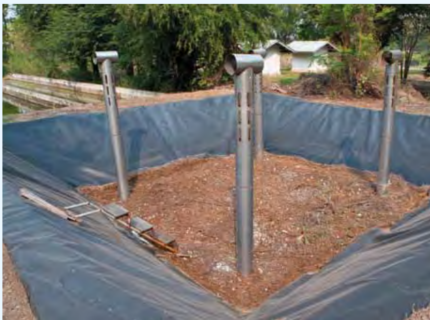
Figure 8.4 A currently out of use pilot-scale drying bed at the Asian Institute of Technology (AIT), showing ventilation pipes (photo: Linda Strande).
