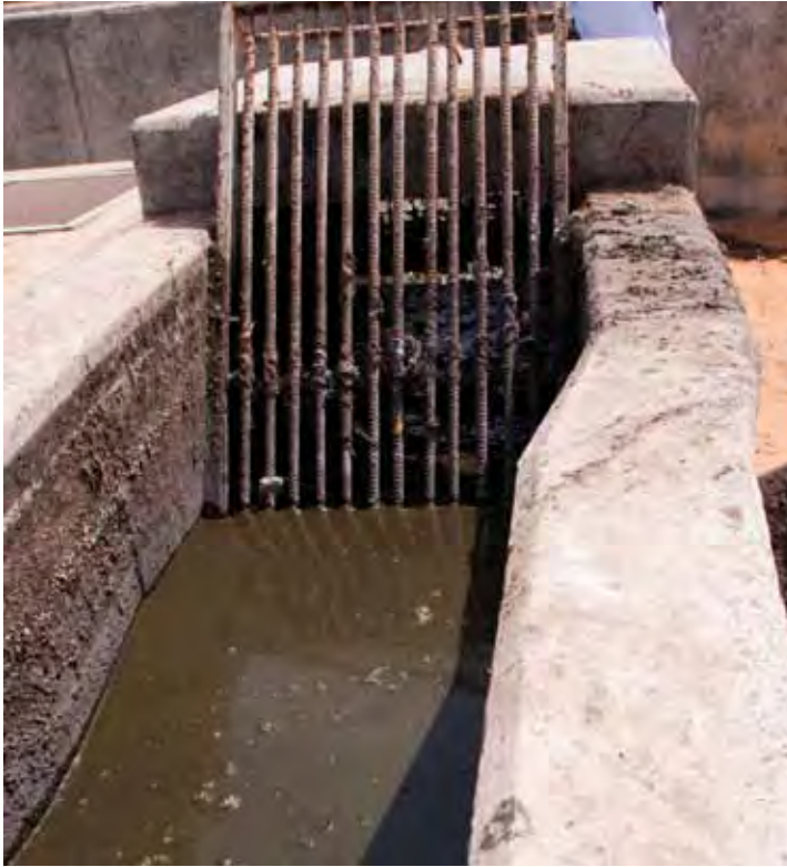
Figure 3.6 Bar screen at Niayes faecal sludge treatment plant, Dakar, Senegal (photo: Linda Strande).
