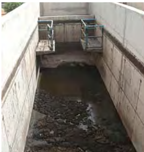
Figure 6.6 Settling-thickening tank of Rufisque showing the scum layer (photo: SANDEC).
